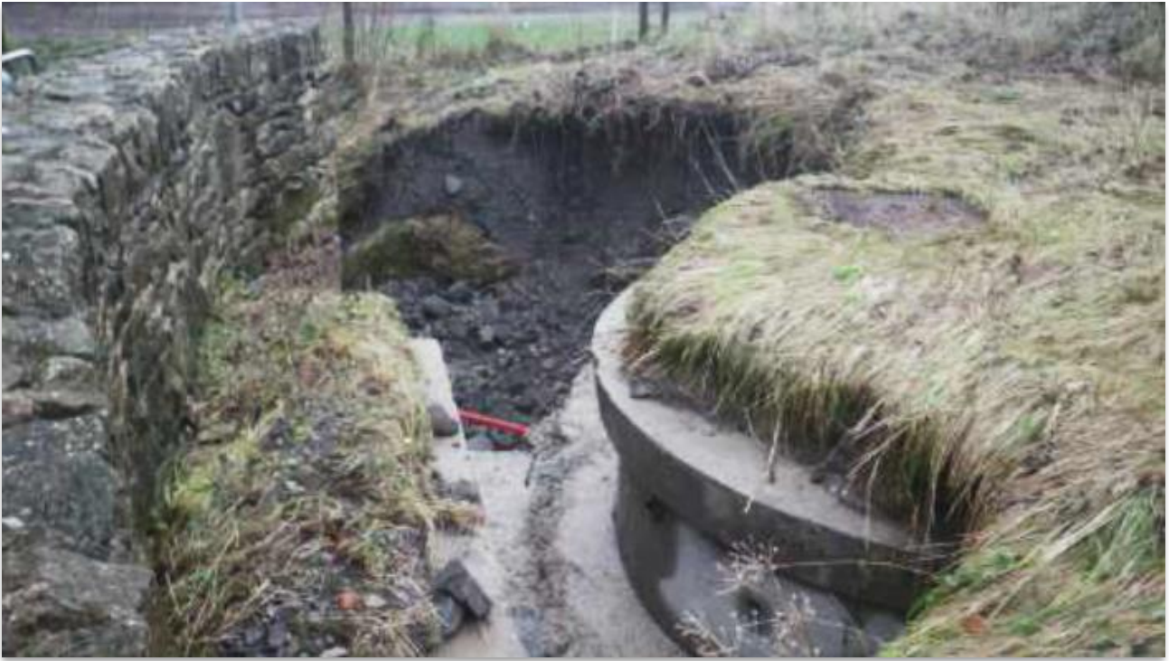
Figure 21: Scour damage to rear of outfall structure upstream of Stock Beck FSB
