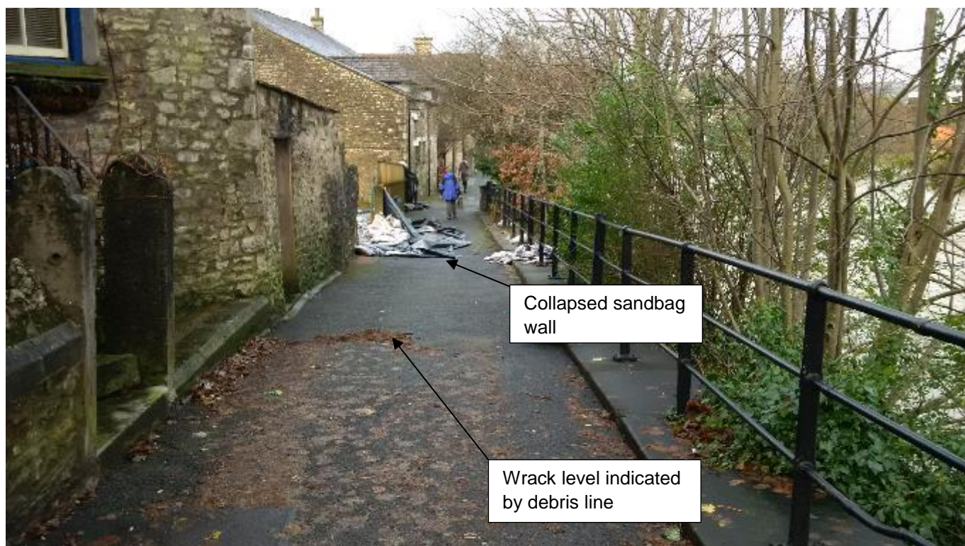
Figure 26: Wrack level on the riverside path at Benson Green, adjacent to Victoria Bridge. Note the sandbag wall which has collapsed towards the river.
