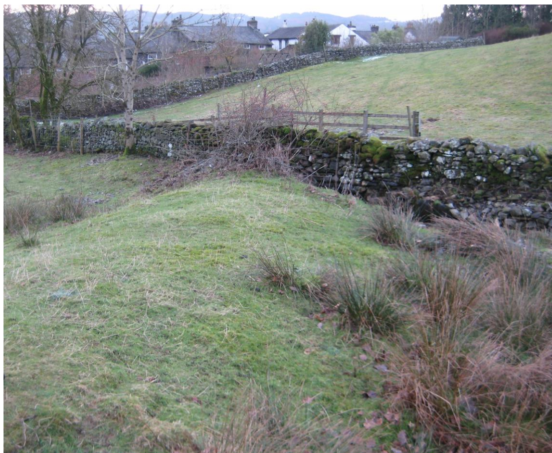
Figure 5 – Short length of raised ground next to the Bell Beck culvert inlet
