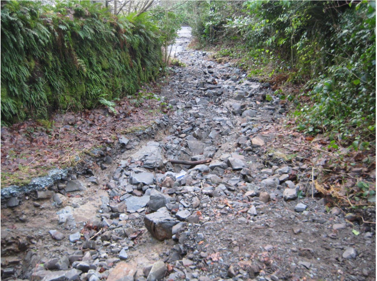
Figure 11 – Damage on Rough Lane, looking downstream towards the A592
