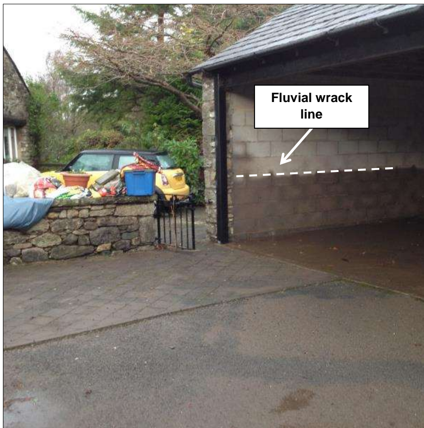
Figure 2: Wrack line in an external garage on the left bank of the River Bela at Parsonage Fold
