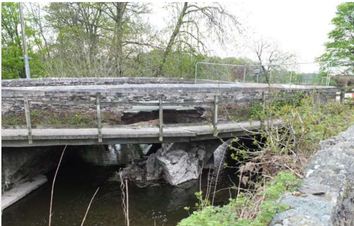
Figure 7: Structural damage to Gowan Bridge
