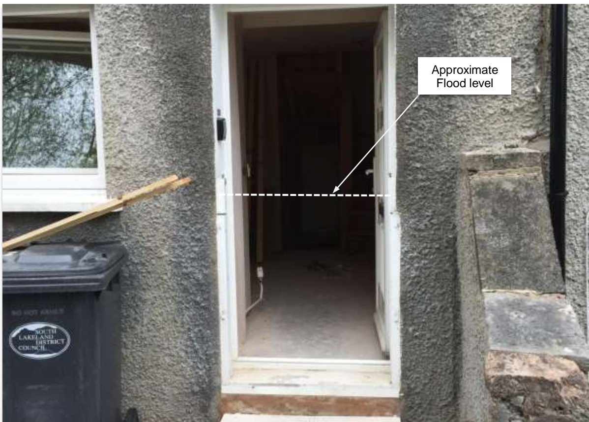
Figure 13: Affected property on Bridge Street, Burneside
