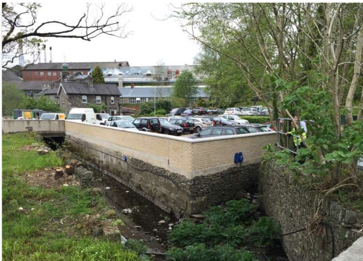
Figure 20: Properties on Bridge Street and New Street flooded initially as a result of water being trapped on the 'dry' side of the flood defence wall
