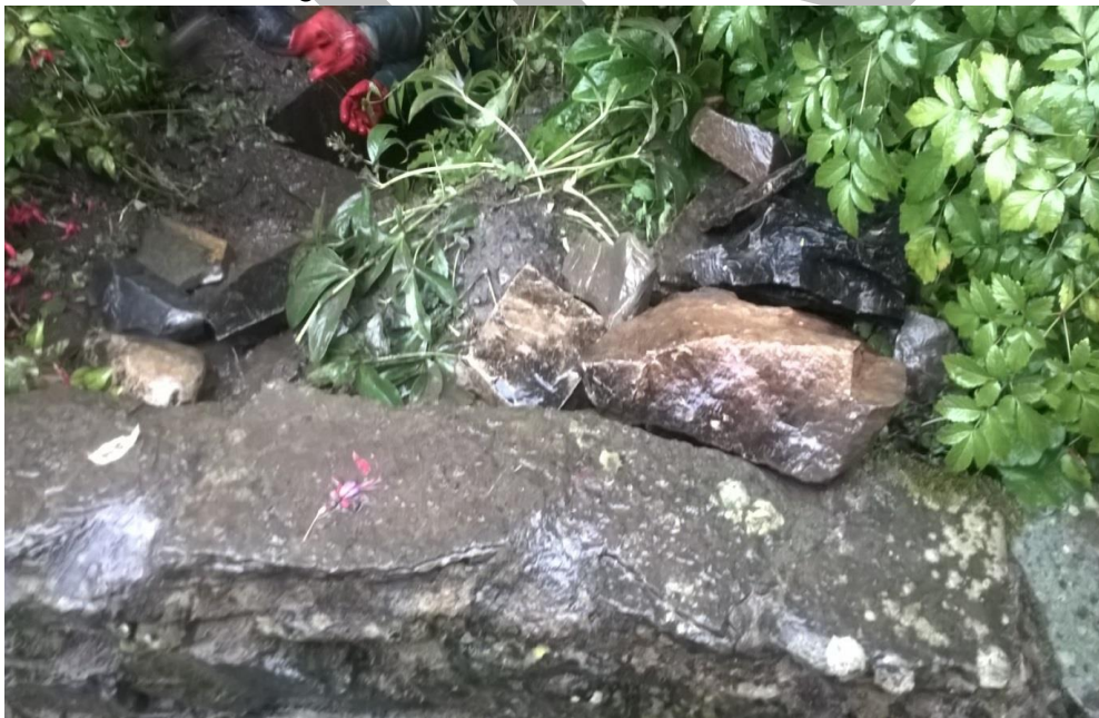
Image A: Debris removed from culvert by hand located in the Garden of “The Nook”
