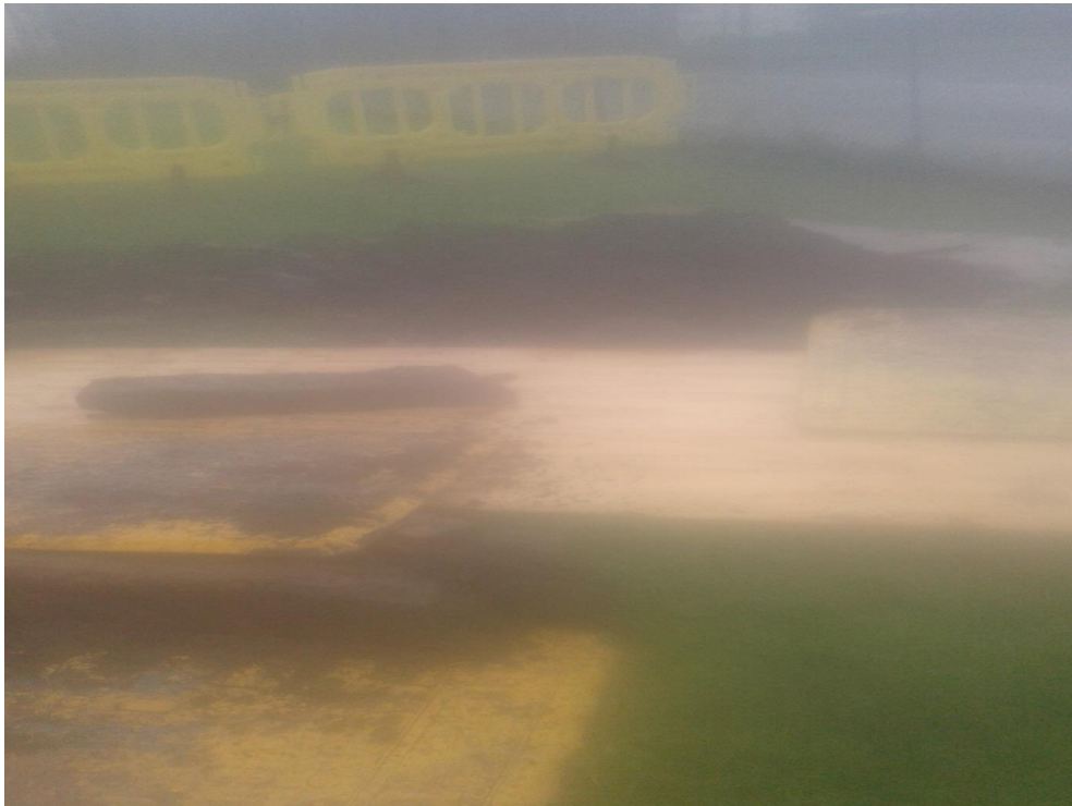
Image B: Shows the location of access excavation 2 in the grass verge opposite Guldrey Terrace.
