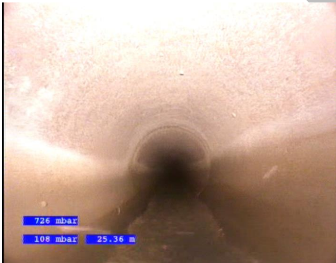
Image F: Shows the 450mm pipe through the new build development to Guldrey Fold
