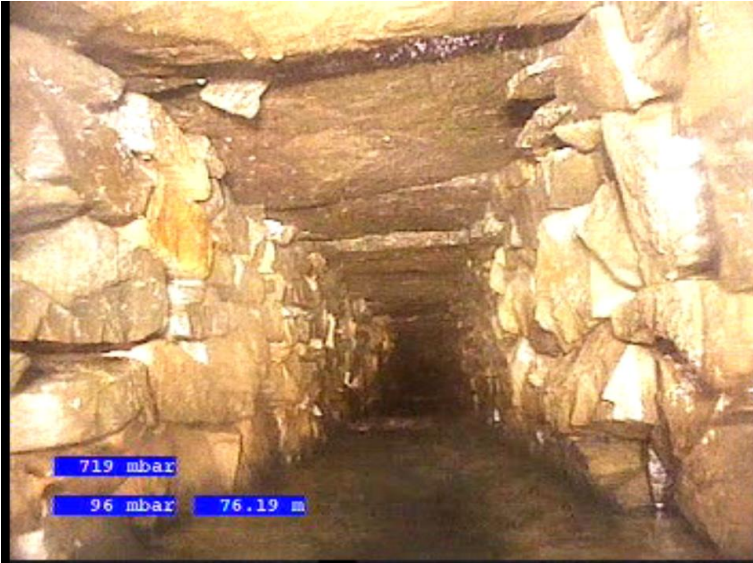
Image G: Shows the downstream section of the box culvert at the end of Guldrey Terrace before discharge into the 450mm pipe
