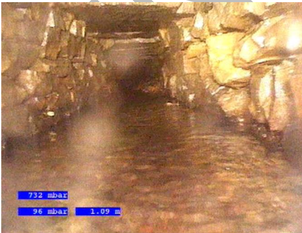
Image C: Condition of the culvert after removal of debris, Note debris bank in the distance.
