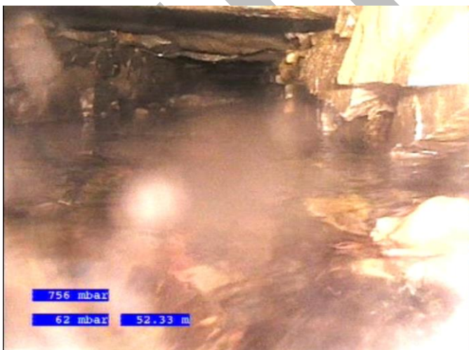
Image D: Indication of culvert capacity loss during Sapphire works
