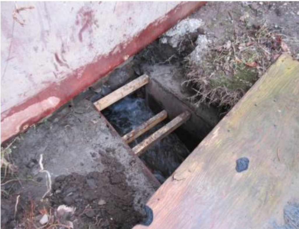
Image 6 – Indicates the location in the rear of The Nook where the watercourse had forced its way out of the old stone culvert. The image was taken by residents after the event and after works had been done to repair the culvert wall collapse.
