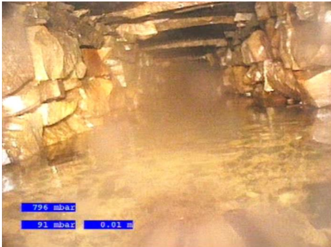
Image E: Indication of the improved capacity following works undertaken by Sapphire
