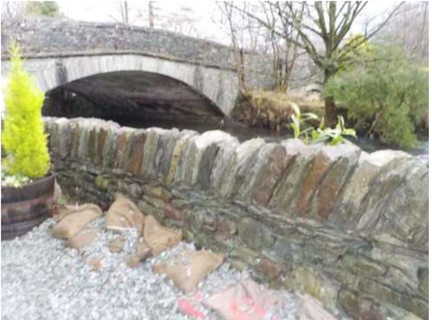
Figure 9 – A privately-owned, informal flood defence downstream of White Bridge (photo taken looking upstream). The wall apparently overtopped during the December 2015 flooding. (Note that the arch in White Bridge just visible on the right of the photo is for a mill race and watercourse that flows from Greatcross Cottages).
