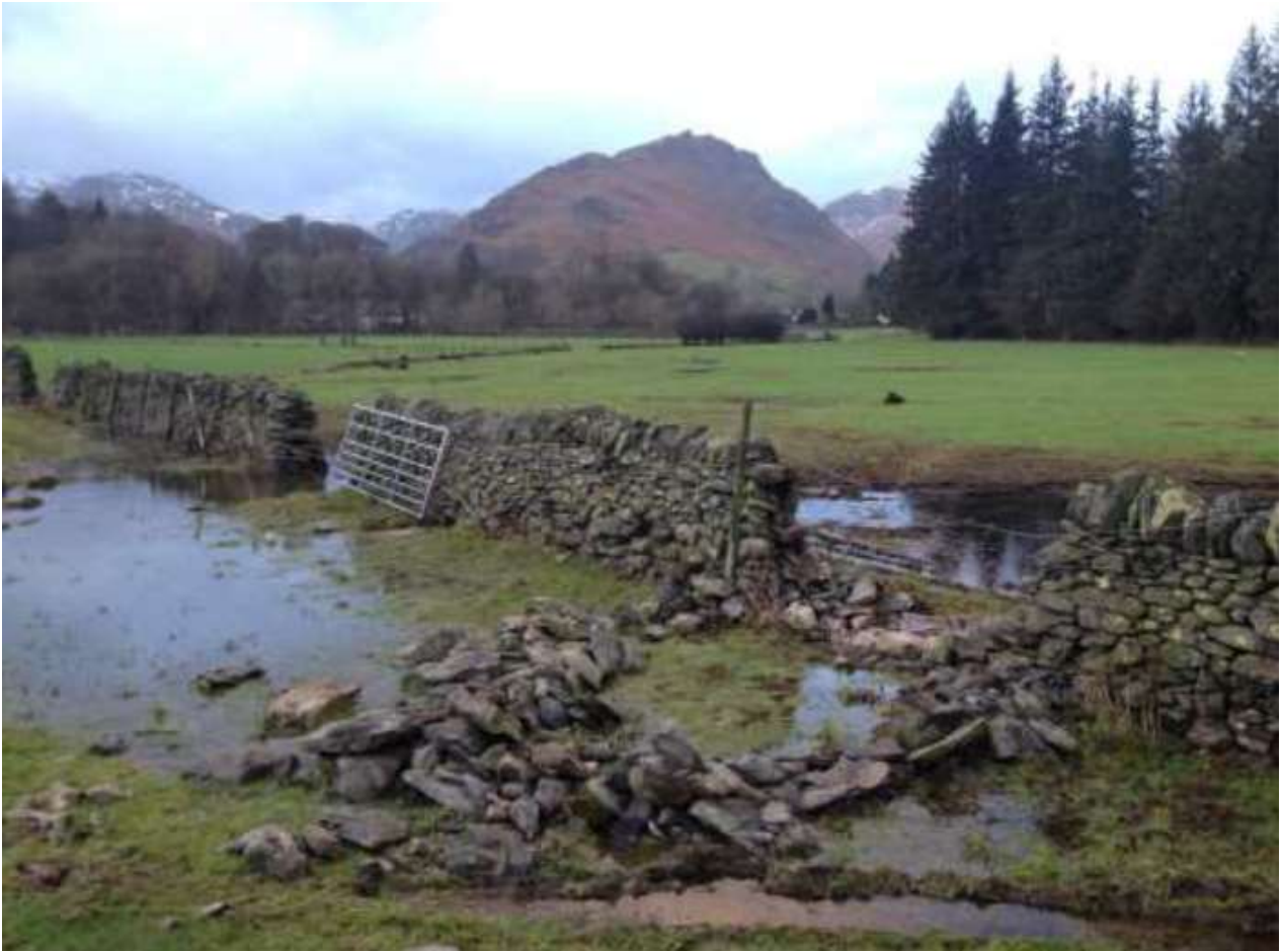
Figure 18 – Damage to dry stone walls on left bank floodplain of the River Rothay due to flood water.
