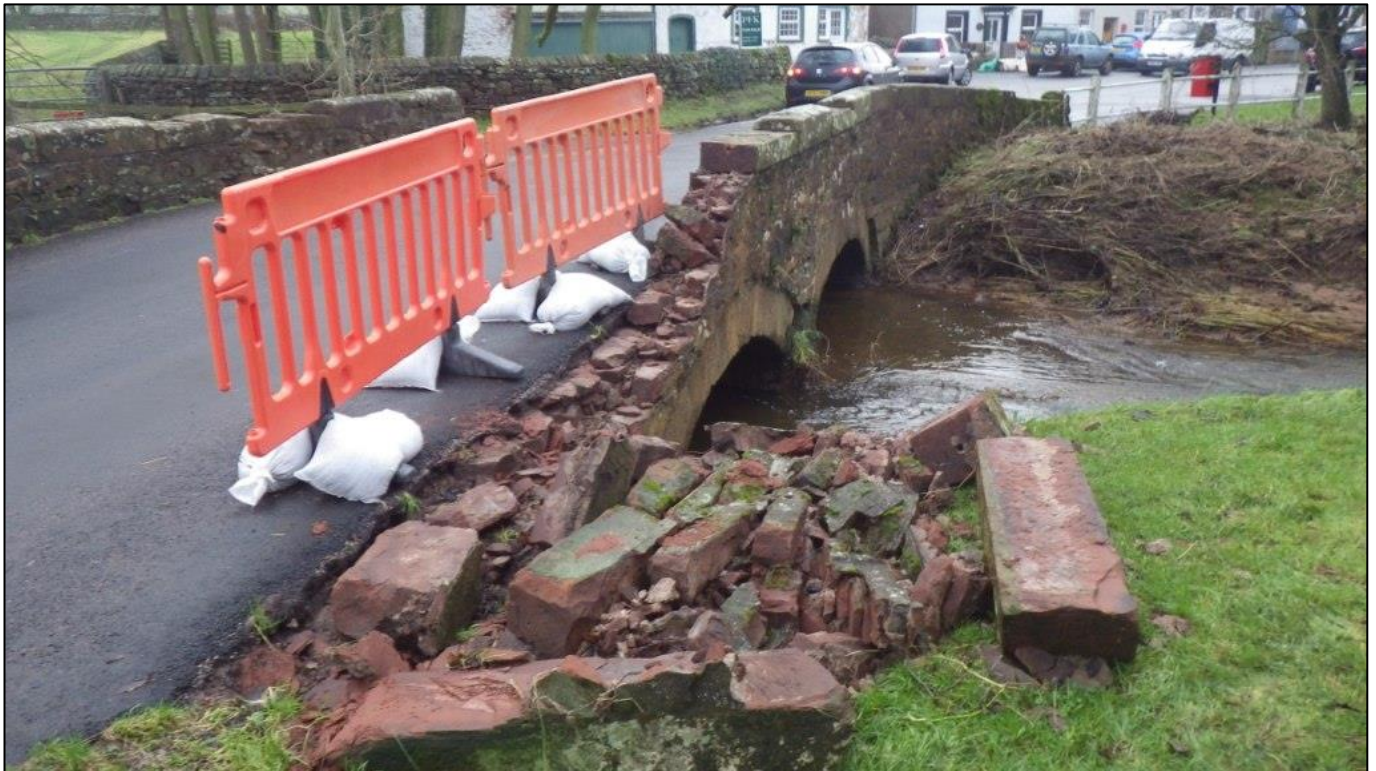
Photograph 4: Flood Damage on Warcop Bridge over the Lowgill Beck, looking south 15 th December 2015, no timestamp
