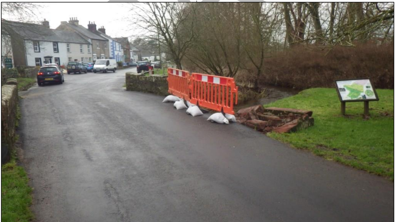
Photograph 3: Extent of damage on Warcop Bridge looking downstream 5 th December 2015, no timestamp
