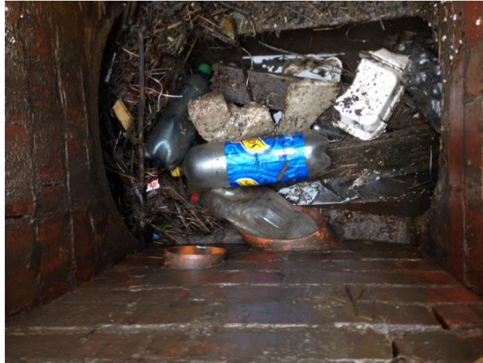
Photograph 3: Debris in one of the manholes in the culvert
