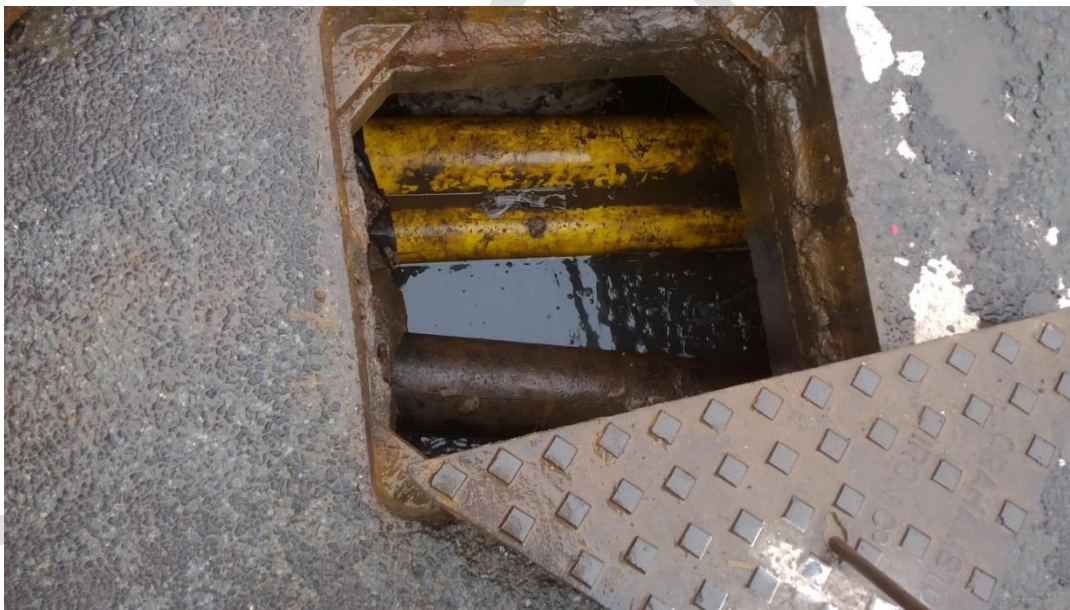
Photographs 4: Services through the drainage systems
