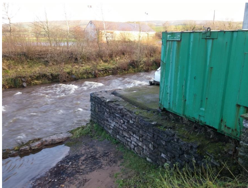
Photograph 9: River wall that was almost over-topped.
