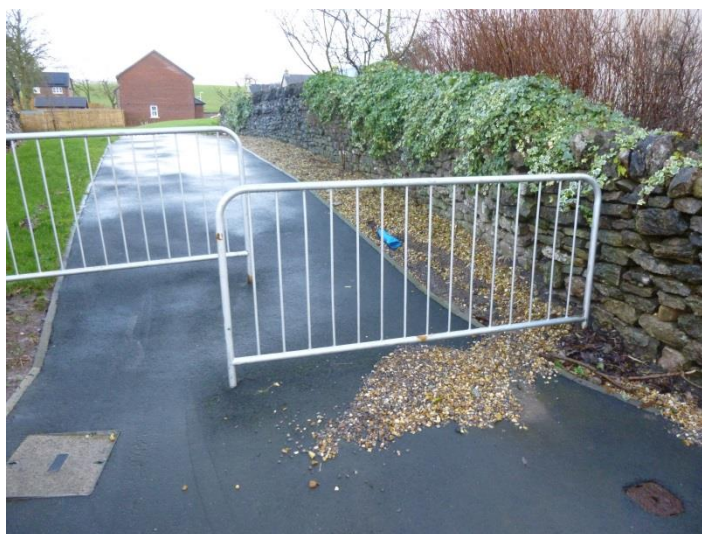
Photograph 6: Damage caused by overwhelming of drainage system through Birkbeck Gardens
