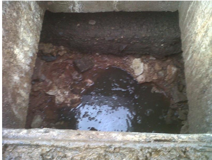
Photograph 8: Indication of silt build up within the Croglam Beck culvert
