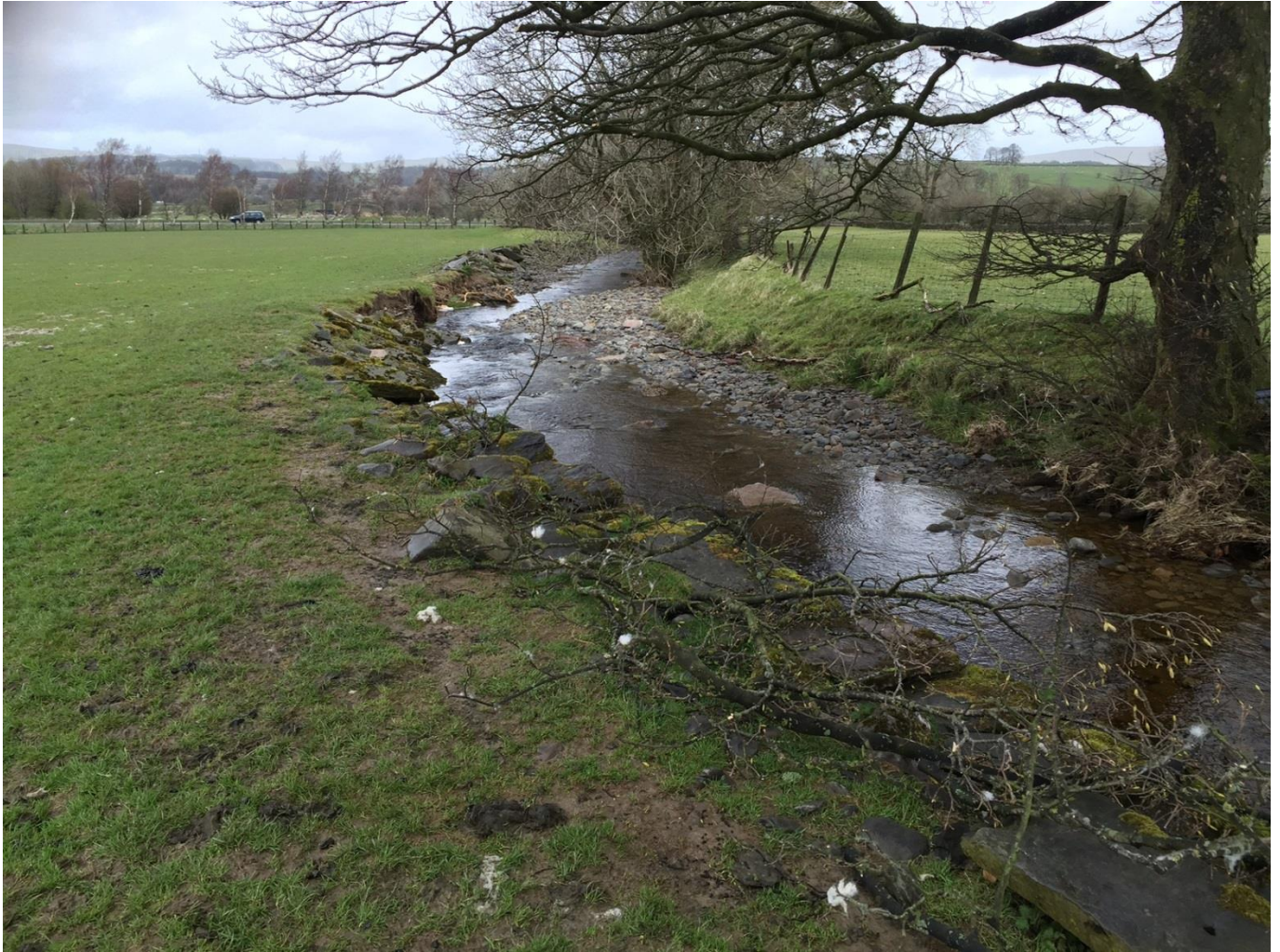
Photograph 10: Raised embankment on the eastern bank of Tebay Gill Beck downstream of the minor road bridge
