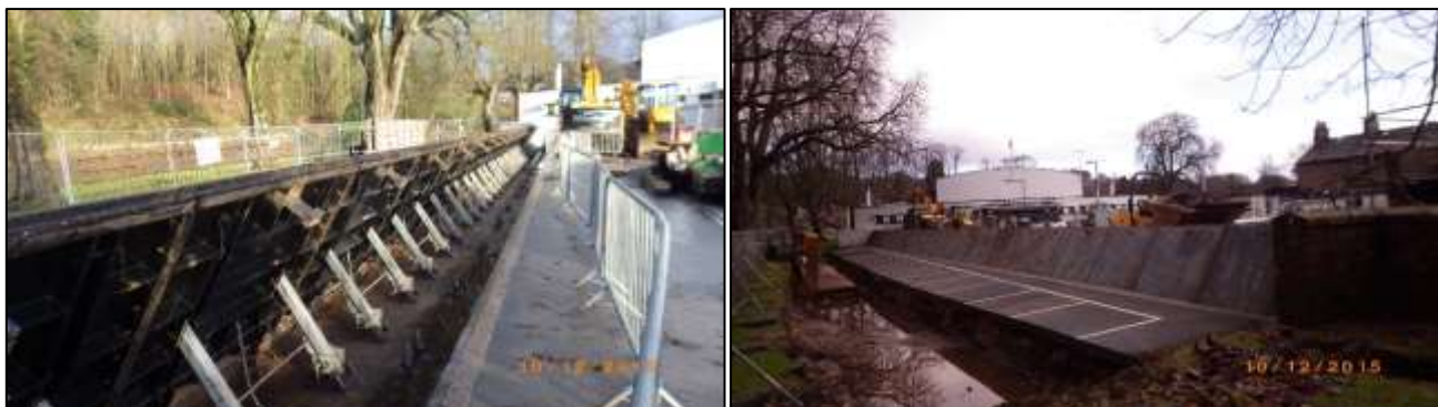
Photographs 19 and 20: After flood peak - Flood Barrier in Operation at Appleby Leisure Centre
