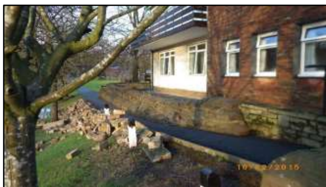
Photograph 23: Collapsed flood wall at Edenside Care Home
