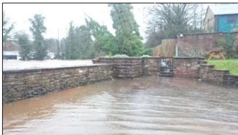
Photograph 13: Stone wall on the left bank - water seeping through 13:22 hrs 5 th Dec. '16
