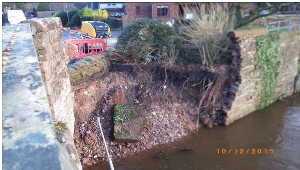
Photograph 9: Left bank retaining wall collapsed
