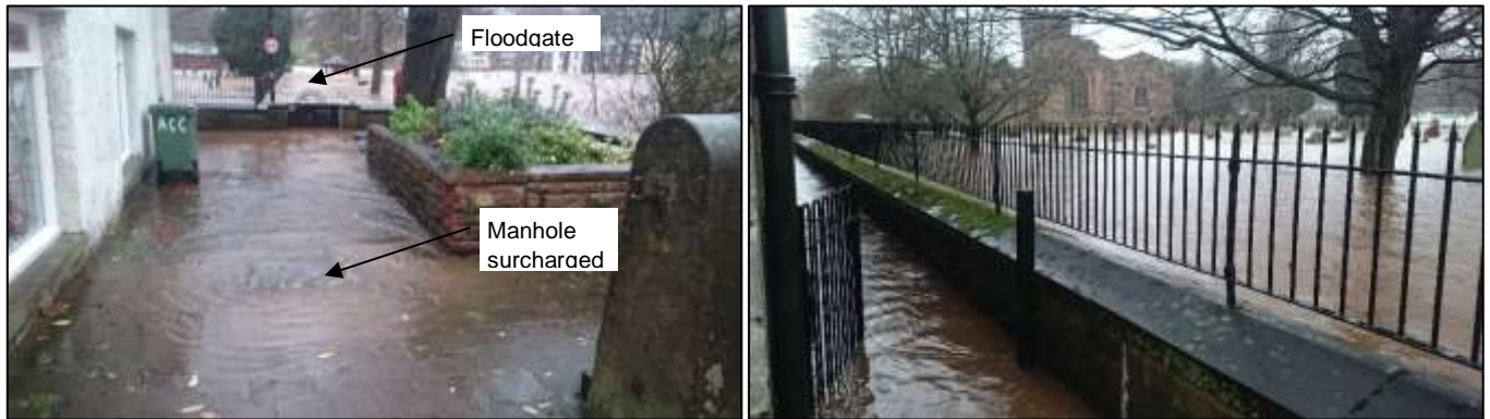
Photographs 14 and 15: Surcharged manhole behind the flood defence 13:40 5 th Dec. '15
