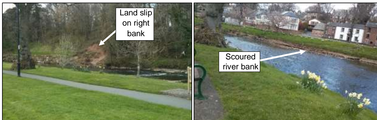
Photographs 26 (left) and 27 (right): Land Slip and Scour on Right Bank
