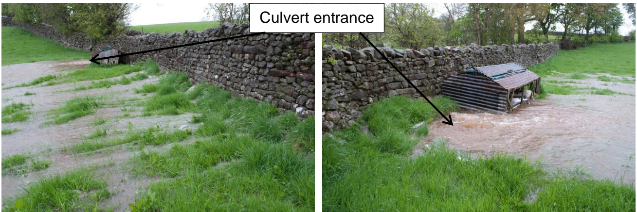
Photographs 7 & 8: Floodwater flowing through wall from bridleyway shown in photograph 6.
