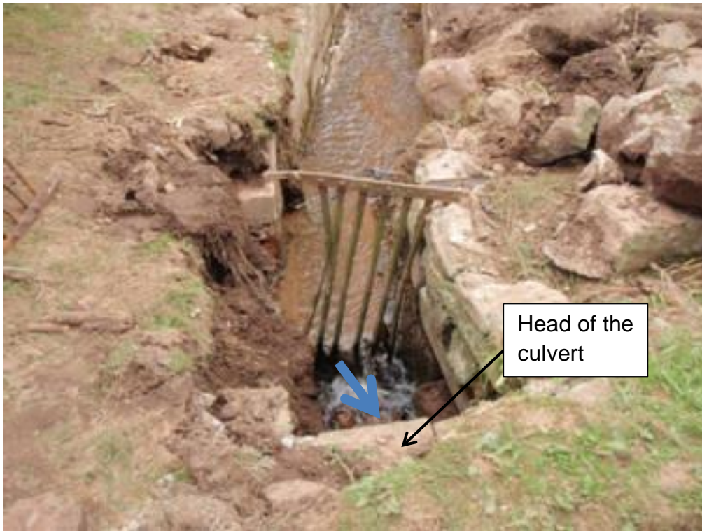
Photograph 5: Damage to culvert entrance following 28 th June 2012 event
