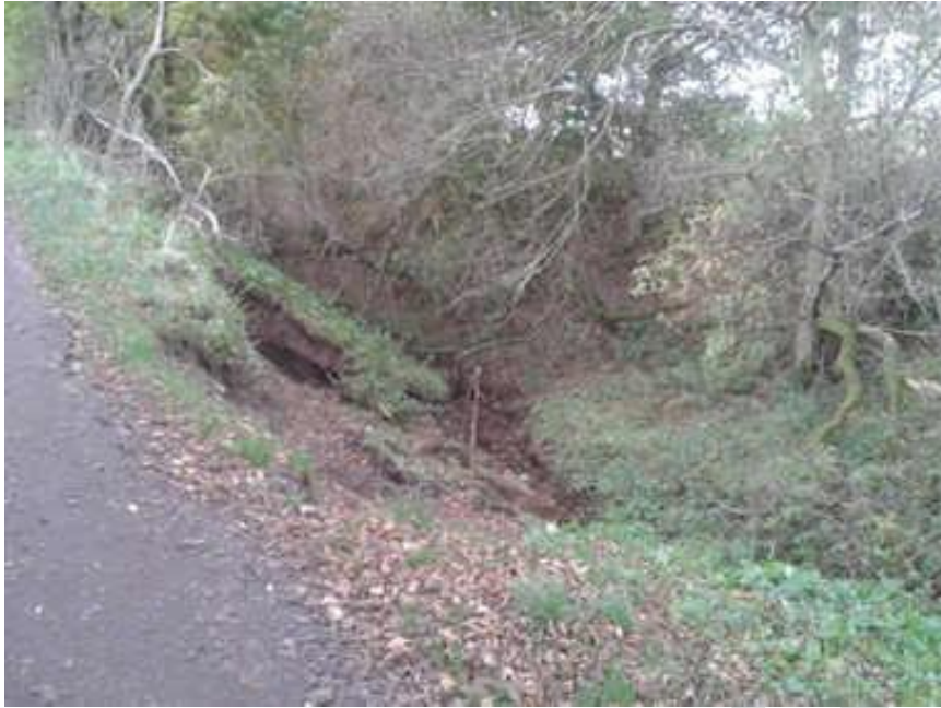
Photograph 1: Landslip near the junction of Green Rigg track and Ormthwaite Road
