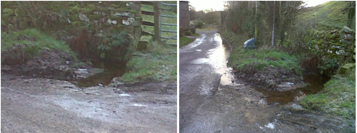
Photograph 9 & 10: Evidence of blocked drainage pipe near Quarry Farm
