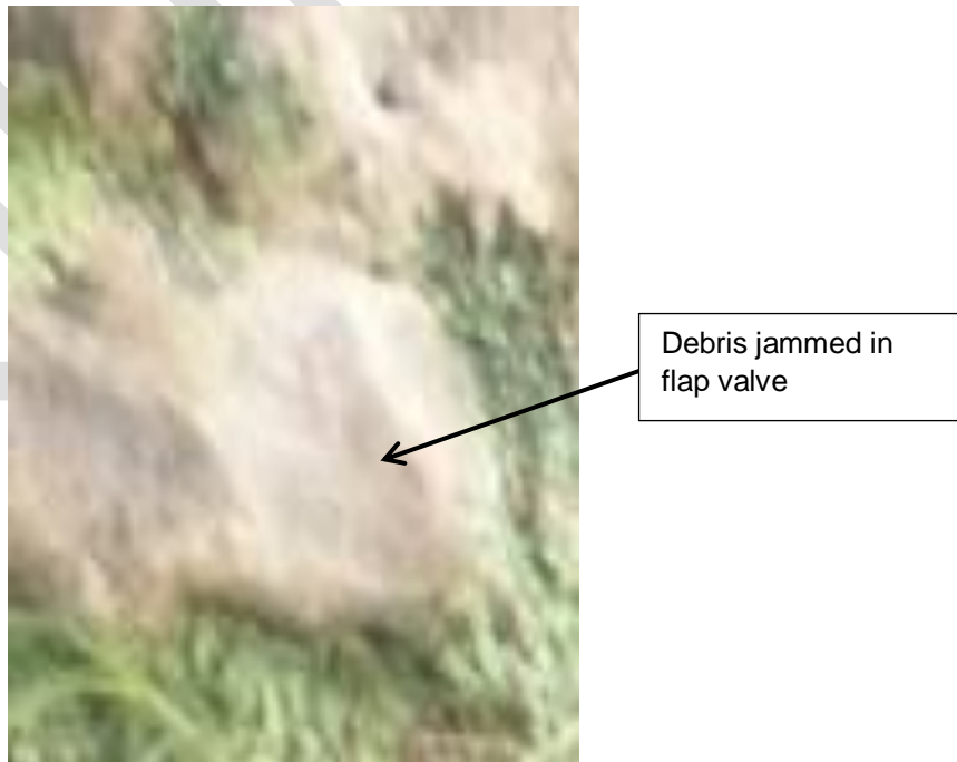
Photograph 3: Debris jammed in flap valve on surface water outfall Photograph courtesy of the EA
