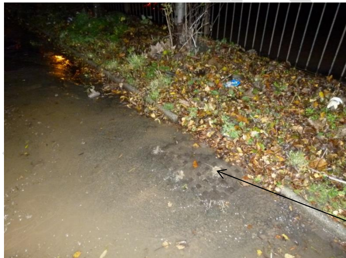
Flood water surcharging from gullies and manholes
