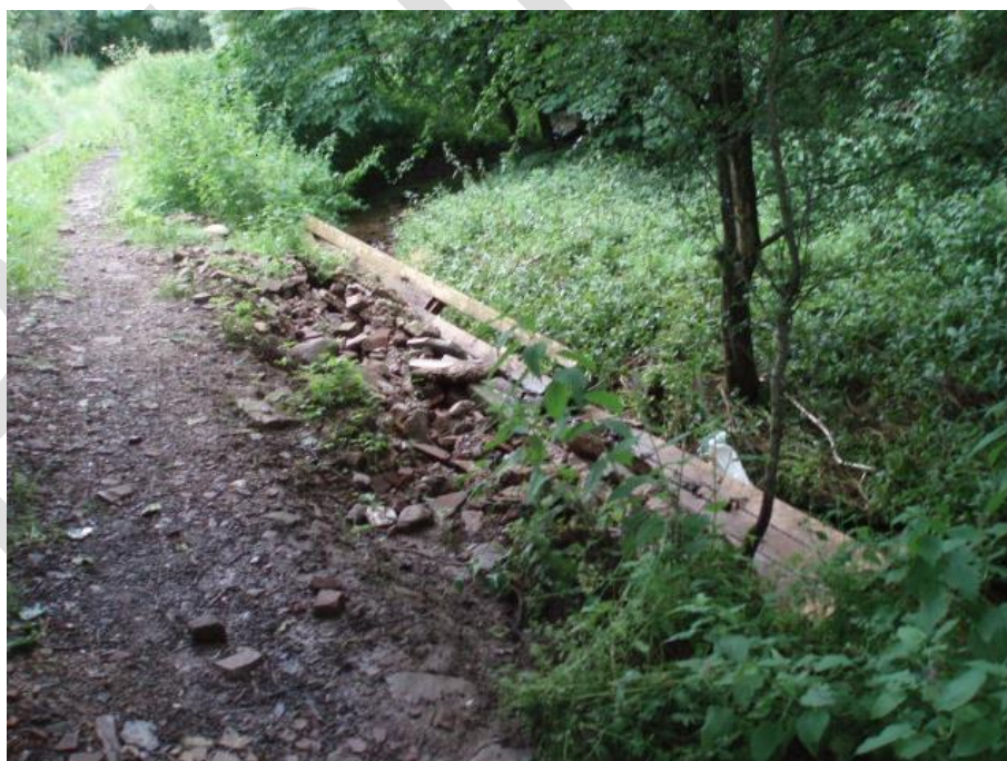
Photograph 1: Erosion and damage caused to Cumrew Beck upstream of Cumrew Village
