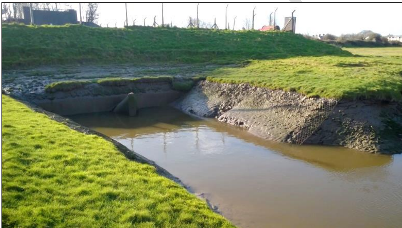
Photograph 1: Duckbill valve at King Street Pumping Station
