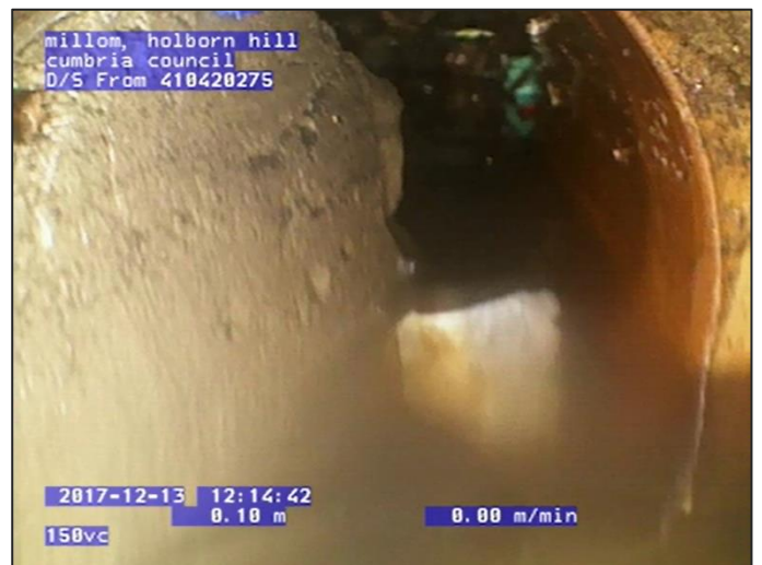
Figure 27: Standing water in damaged highway gully
