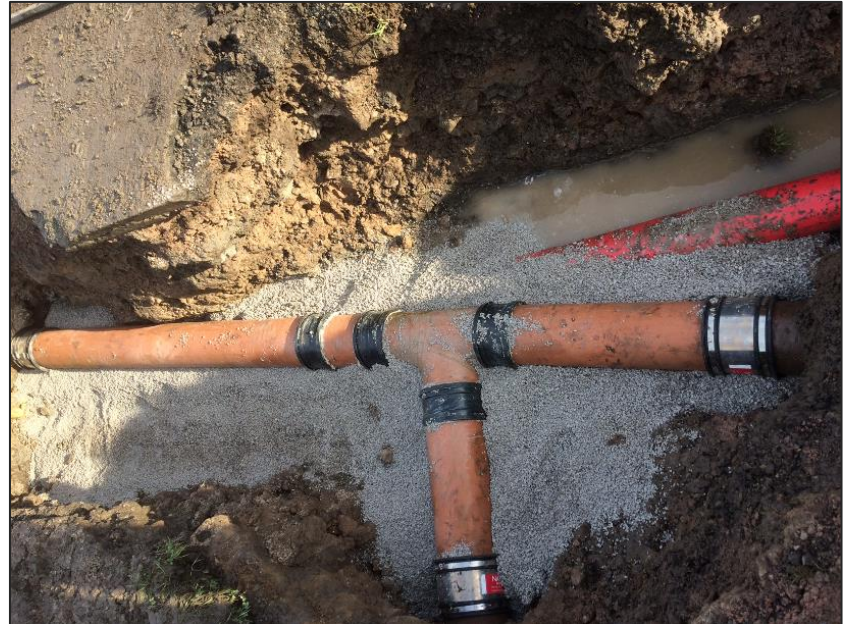
Photograph 2: Highway drainage reinstated on Mainsgate Road. Photo courtesy of Electricity North West
