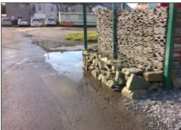
Figure 25 (left): Standing water on collapsed chamber
