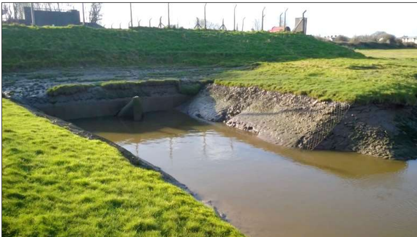
Photograph 1: Duckbill valve at King Street Pumping Station
