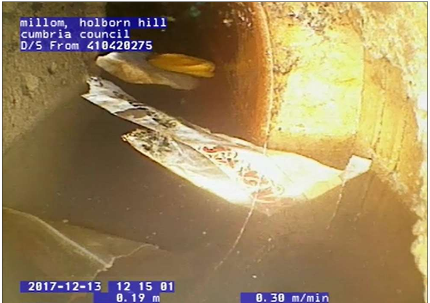
Figure 15: Standing water in damaged highway gully
