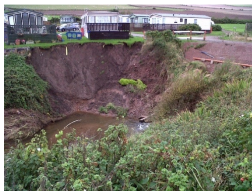
Figure 14. Embankment damage within the caravan park
