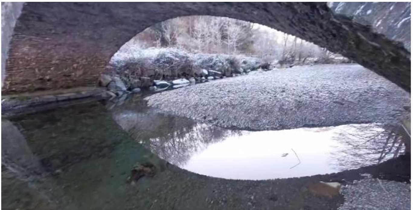
Under Grange Bridge showing gravel deposits
