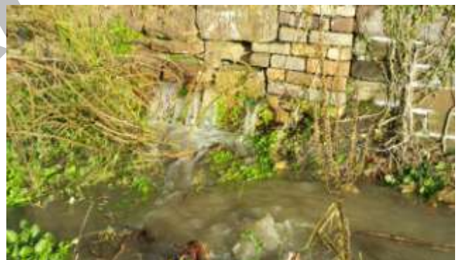
Figure 21 Barepot Reservoir wall leaking
