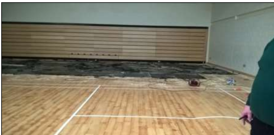
Photograph 9: Nelson Thomlinson School – Sports Hall Flood Damage
