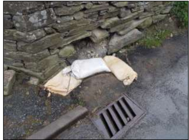
Photograph 16: Improvised surface water flow barrier
