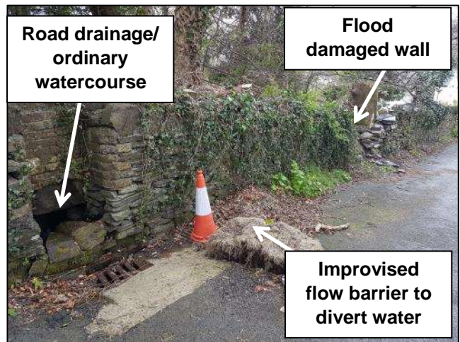
Photograph 14: Flood damaged wall and improvised surface water flow barriers
