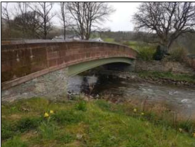
Photograph 17: Looking upstream towards Lorton Bridge from the right bank of the River Cocker
