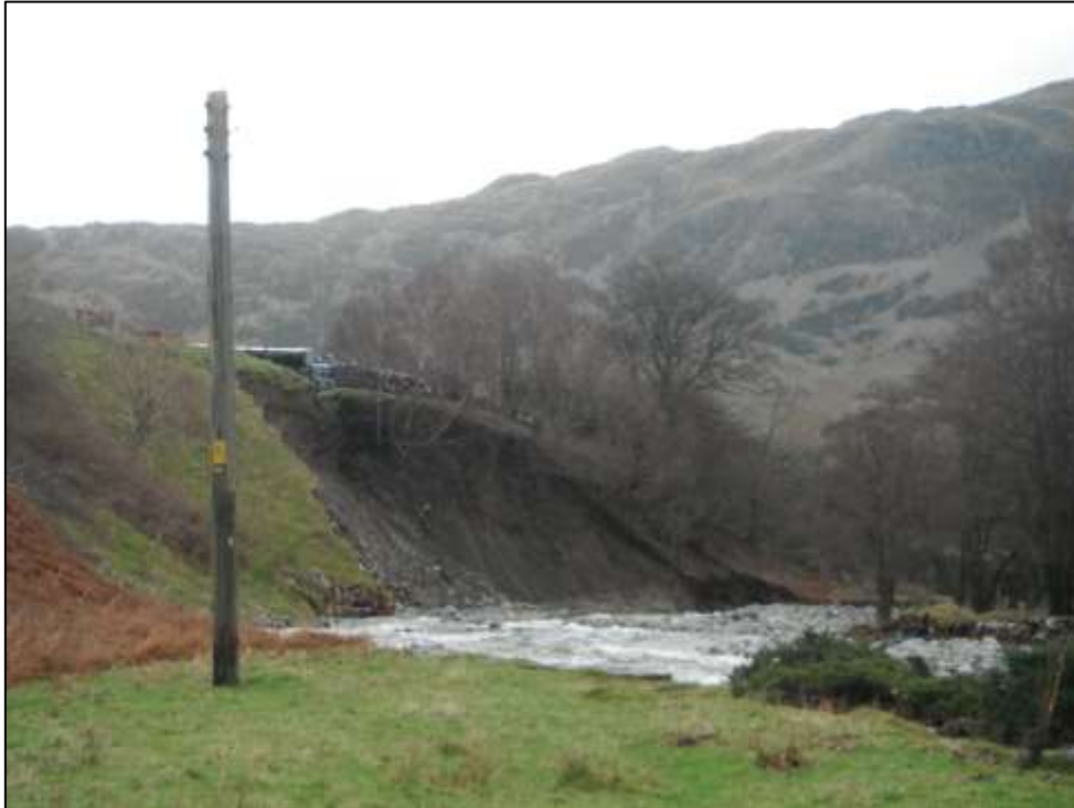
Figure 9-Bank erosion upstream of Glenridding. Date Taken XX/12/2015
