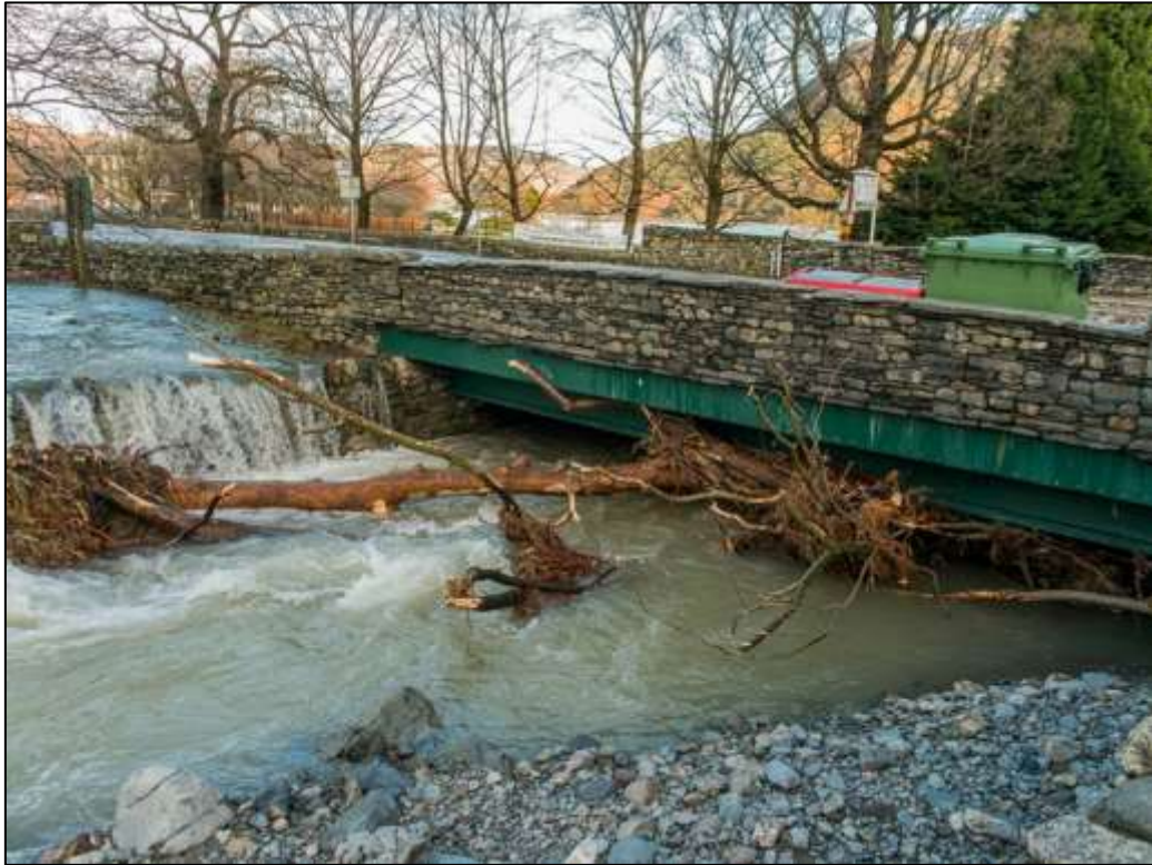
Figure 13-Glenridding Bridge Blocked by debris. Photograph provided by Patterdale Parish Flood Group. Taken XX/12/2015
