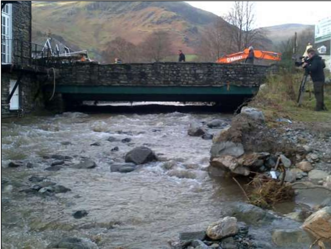
Figure 7-Glenridding Bridge 10 th December 10:49
