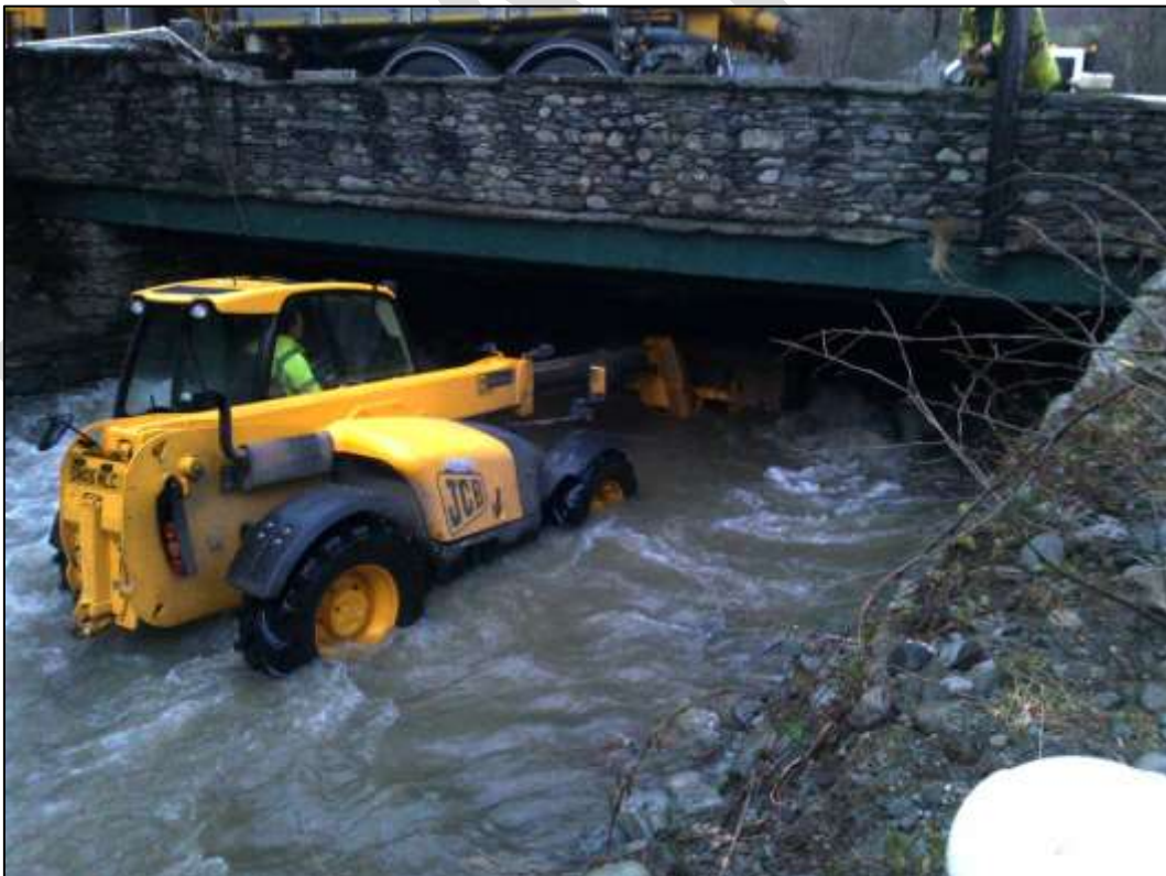
Figure 8-Gravel removal and blockage removal, Glenridding Bridge 11 th December 14:47
