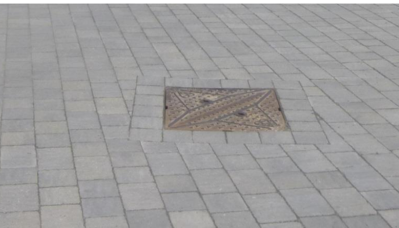
Figure U2: Awkwardly aligned access cover is made apparent through use of setts
